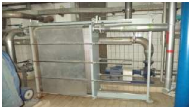
Figure 2 Wort preheater in Tuzla Brewery
